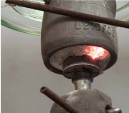
Figure 4 : arc remains outside on a broken glass insulator (also called “stub”)
