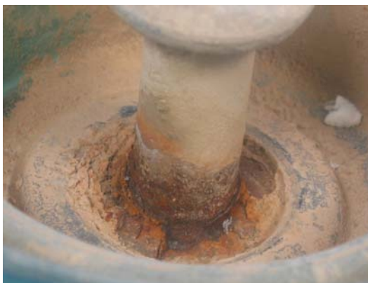
Figure 2: Pin corrosion after more than 20 years in service in severe condition (Iran)
