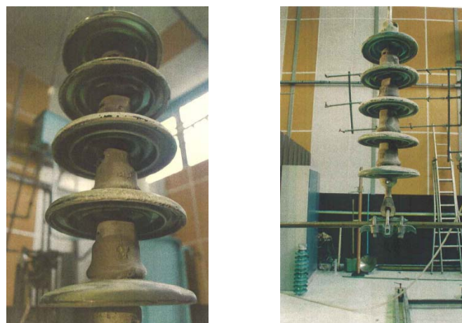
Figure 5 : Electrical type tests on BS1513 insulators after 27 years of service on a 132kV line in Malaysia.
