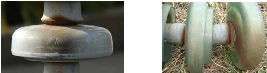
Figure 5: Rust leaching on the surface of the dielectric when the cap is not protected against corrosion.
