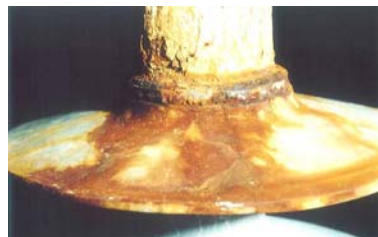
Figure 6: DC corrosion of composite end fitting with heavy rust on the rubber housing
