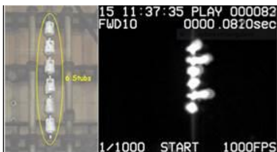
Figure 13: String of stubs during a power arc test showing systematic external arcing.
