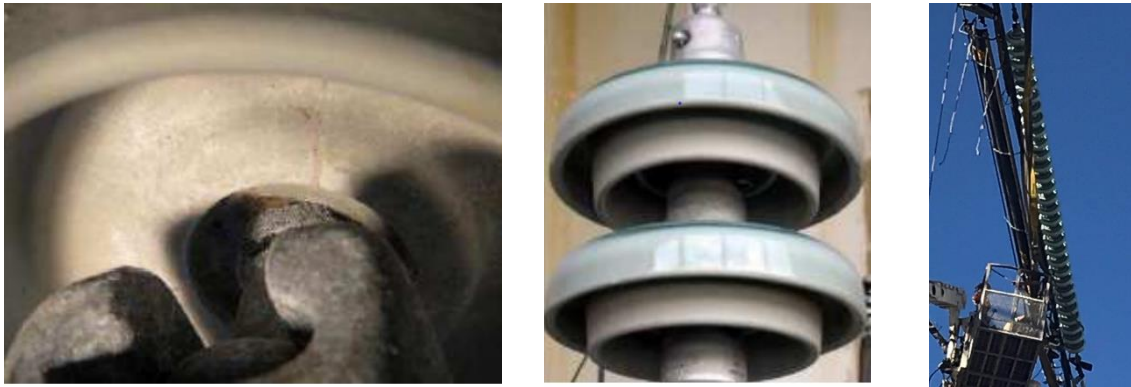
Figure 12: under coated insulators after a 2000h HVDC multi stress ageing test and during installation on a 500kV line
