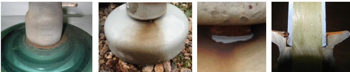
Figure 4: rust at the base of the cap in HVDC applications for glass (left) and porcelain insulators (center). Right: seal degradation and rust on the end fitting of a polymer insulator.
